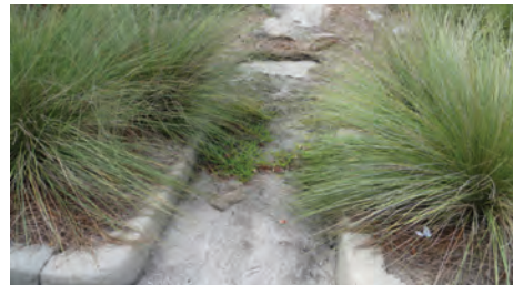
5 INLET STRUCTURE DEBRIS & SEDIMENT
