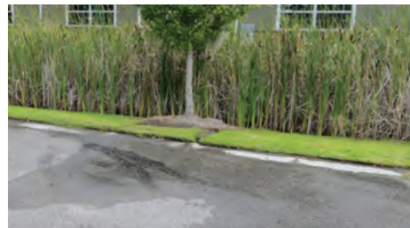
11 EXCESSIVE PONDING (CATTAILS & STAINING)
