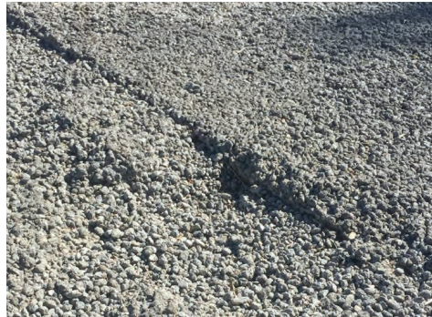
7 CRACKING & 15 RAVELING (POOR)
