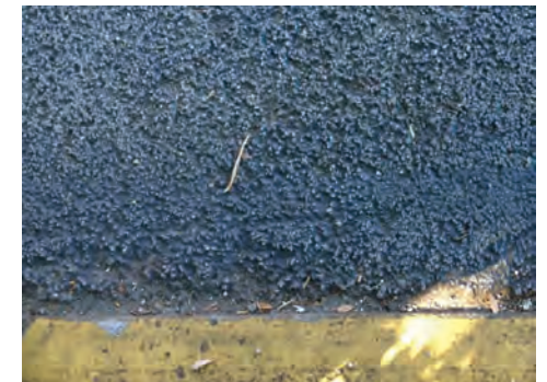
16 SMEARING (POOR) (COVERED WITH ASPHALT SEALER)
