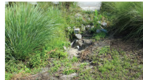
8 INLET EROSION (ROCK PLUNGE POOL)
