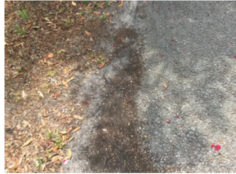
5 UNSTABLE DRAINAGE AREA & 14 DEBRIS (MARGINAL)
