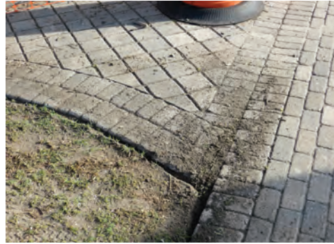
5 UNSTABLE DRAINAGE AREA
