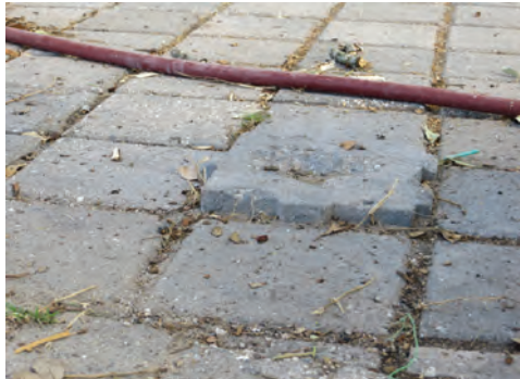
8 STRUCTURAL & 15 SEDIMENT (POOR)
