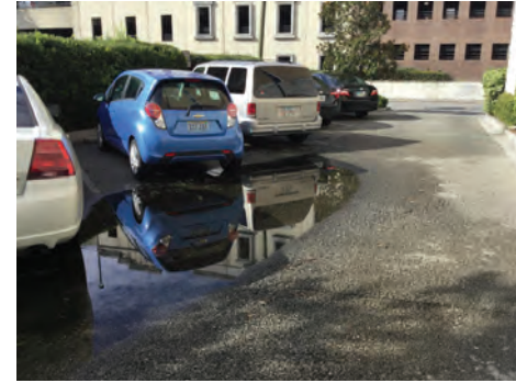
6 PONDING / STANDING WATER
