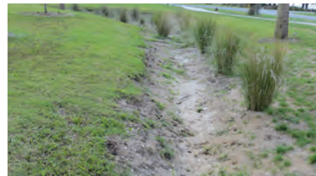
8 INLET EROSION (GRASS CHANNEL)
