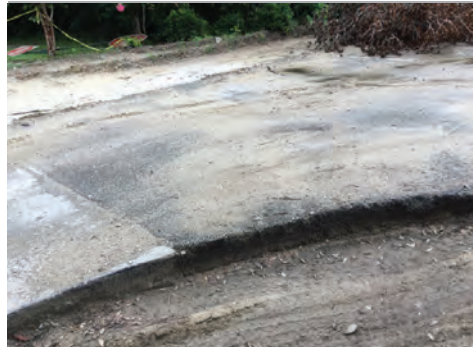
5 UNSTABLE DRAINAGE AREA & 13 SEDIMENT (POOR)
