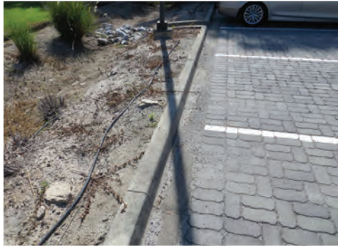
5 UNSTABLE DRAINAGE AREA
